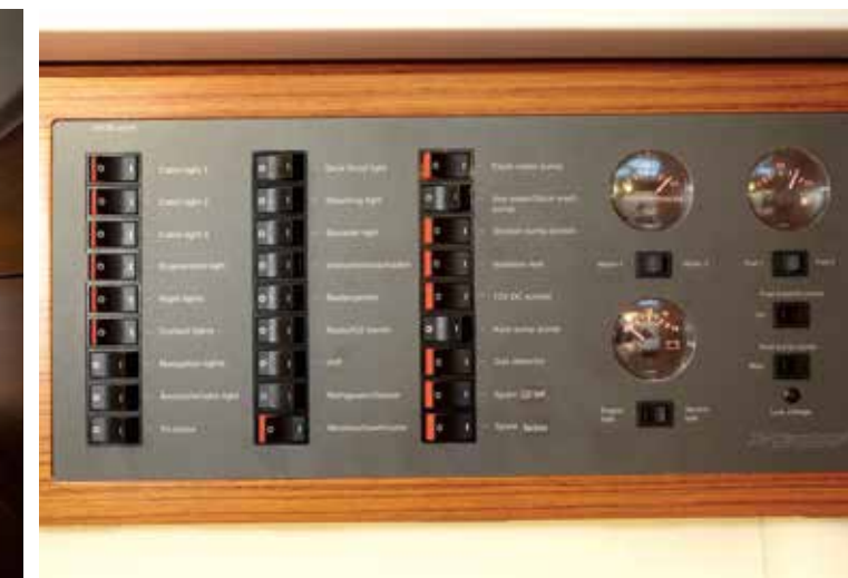
The custom-designed electronic control panel
